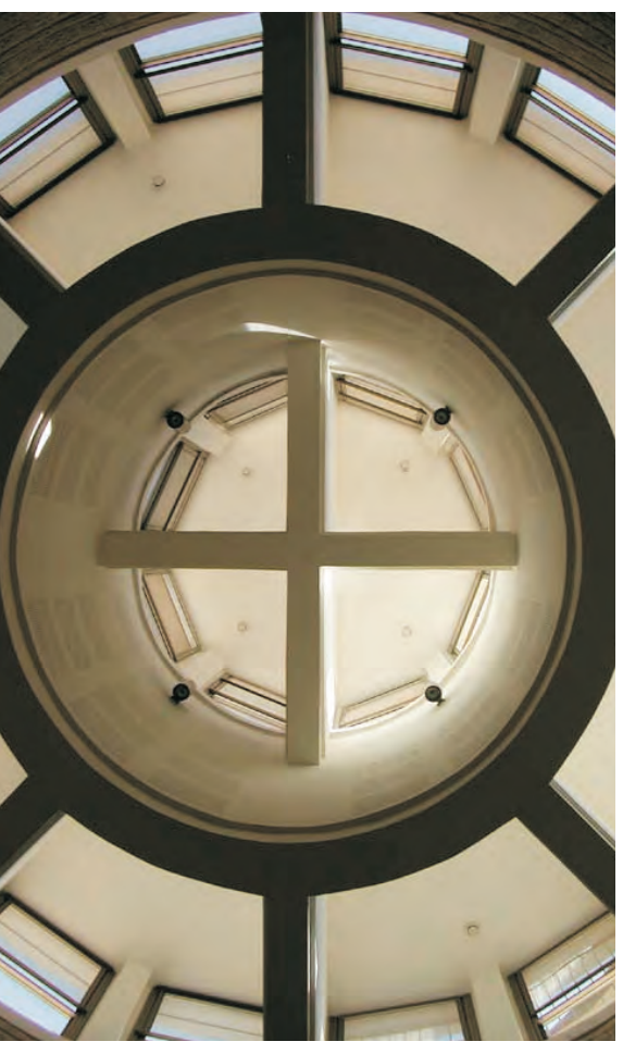
▼ Internal view of the “Cooling Tower”.
